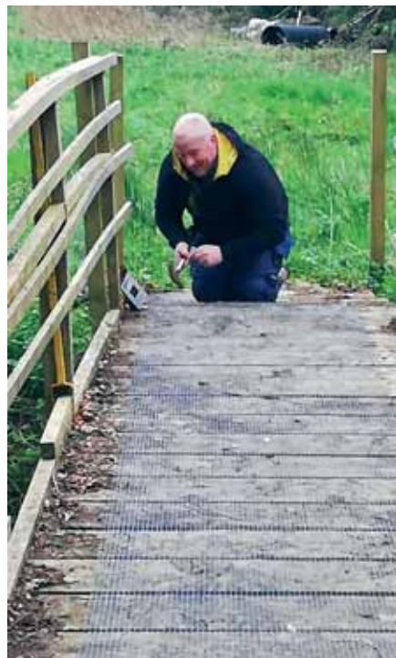
Securing a non slip surface will help in the wetter conditions
