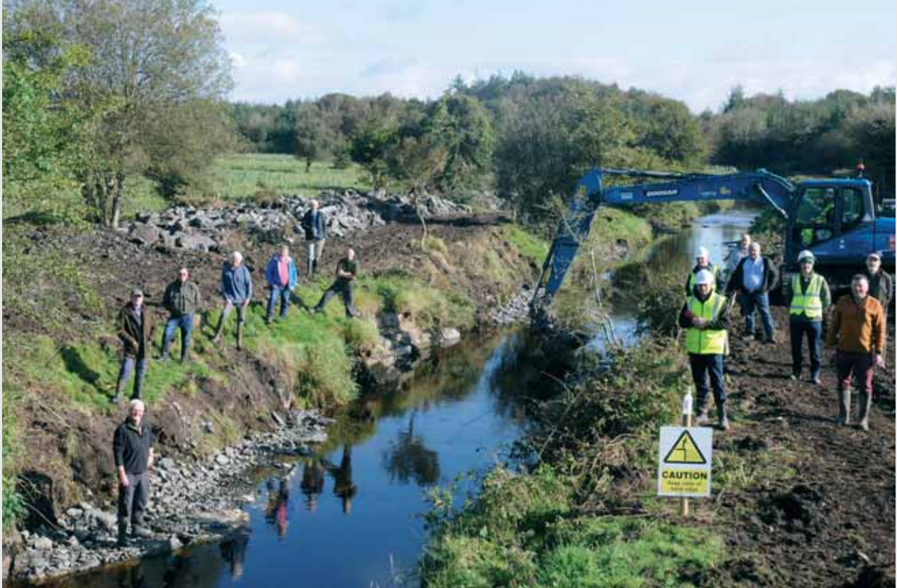
Pat Gorman, Francis O'Donnell and Fintan Gorman from IFI with Local TD Sean Canney, Members of Cairde na Chláir and the Office of Public Works (OPW) at the Abbort River development.
